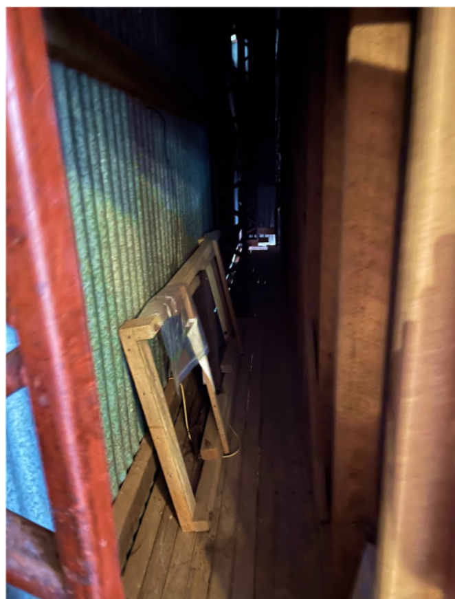
Regular cleaning and monitoring of the crawl space between the timber walls of Baba's Room and the outer walls of Baba's house to assist with pest control and mould prevention.
