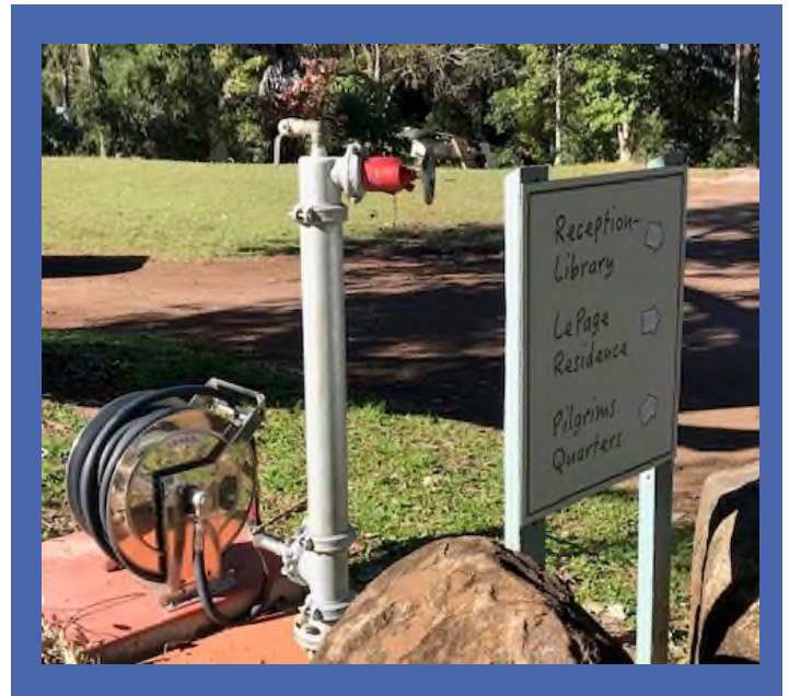
Fire reel and hydrant that the local fire brigade can connect to
